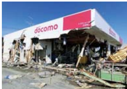
docomo Shop damaged by the earthquake
