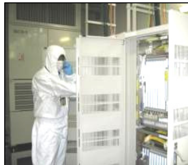
【Apr. 13, 2011】 Replacement of base station transmission lines (Exchange office bldg. in Tomioka, Fukushima)
