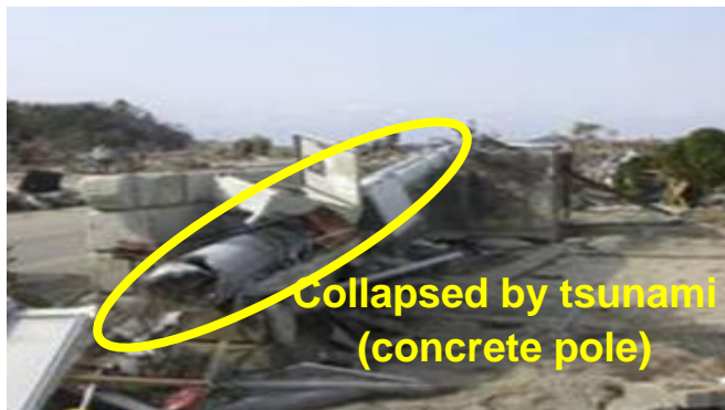
(1) Base station facility (Matsushima-Nobiru, Miyagi Pref.)
